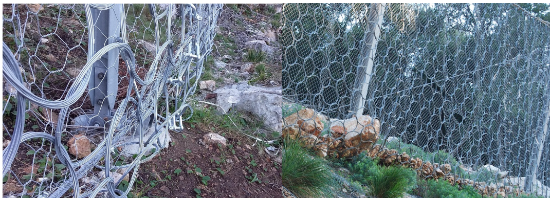
Fig. 2 Pictures of proper elements of a barrier (left) and usual small damages in protection systems (right)
