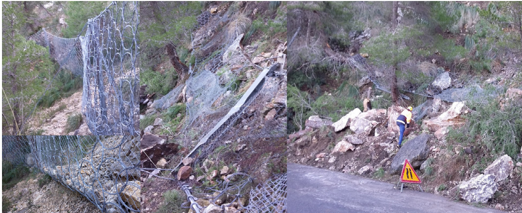
Fig. 3 Pictures of a barrier stated at level 4, installed in 1999, before in 2016 (left) and after it collapsed caused by a rockfall event of 2017-01-31 (mid and right).
