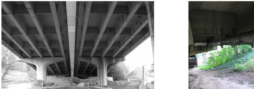
Figure 2: Bridge superstructure (left) and view of a water pipe on girder 1 (right).
