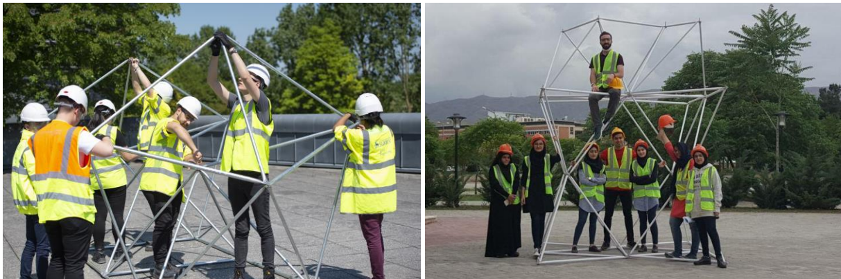
Figure 1 Left: Surrey students assembling the structure designed Mexican students, Guildford, UK. Right: Iranian students after the assembly of the structure designed by Surrey students, Mashhad, Iran.
