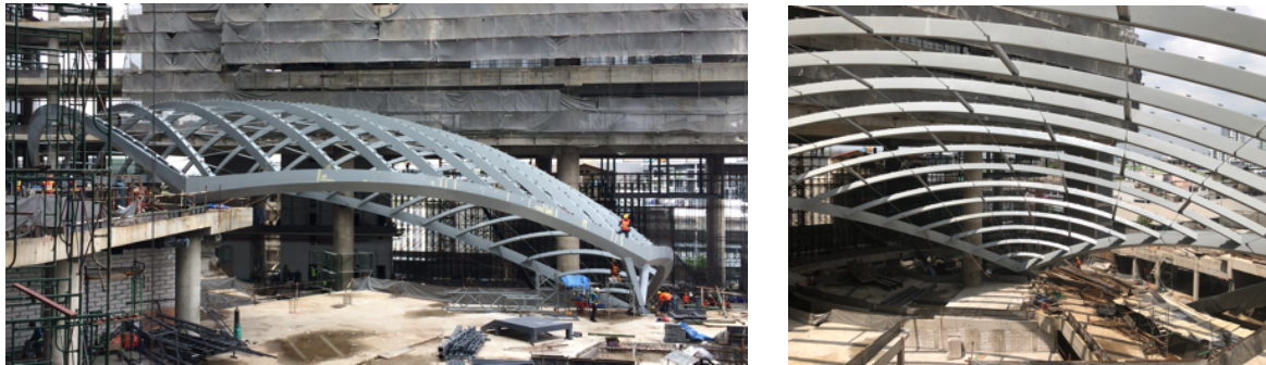
Figure 1. Left: View of the roof under construction. Right: Inside of the roof during construction
