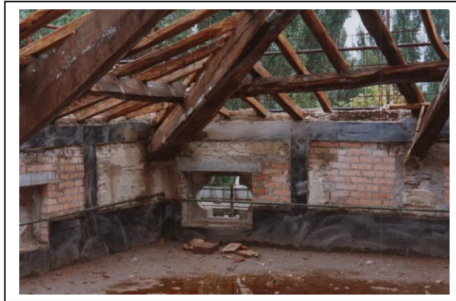
Fig.24- Example of building complete belting ( inside and outside ) , at Villa Bertani- Reggio Emilia damaged by earth quake of 1996 , using thermo welded Betontex unidirectional carbon reinforces.
