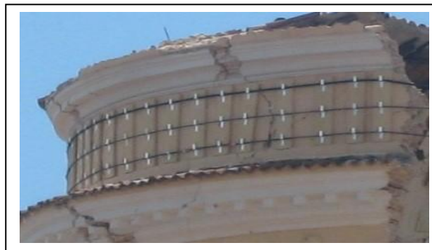
Fig.9. Application of Betontex Aramid Tie 85 HM on the tambour of “Anime Sante” Cathedral, L’Aquila, damaged by earthquake of 2009. The Tambour was put in security to proceed with further works.
