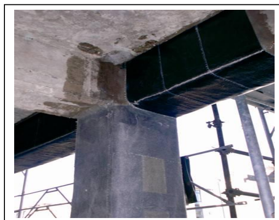
Fig.23- Example of old concrete rehabilitation using thermo welded Betontex unidirectional carbon reinforces.
