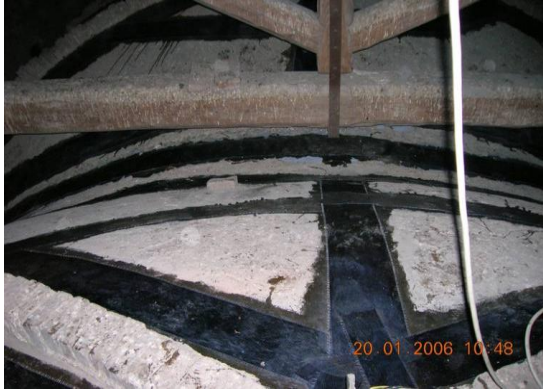
Fig.21- Example of extrados vaults reinforcement by carbon fibres tapes, (S. Giorgio Church, near Bologna-Italy)
