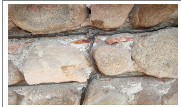
Fig.10. Historical City Walls in stones ( Bassano- Italy), reinforced with hybrid aramid – carbon fibres cable, prestressed and impregnated with epoxy resins. Courses among stones will be filled by traditional mortar.
