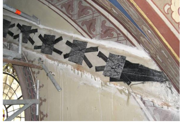
Fig.22- Example of walls reinforcement using Ar-dix connectors, at Alba Cathedral in Cuneo- Italy.
