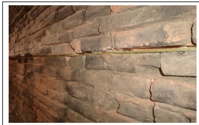
Fig.11. Bricks walls reinforced with carbon fibres cable coated with aramid fibres, prestressed and impregnated with epoxy resins. Courses among bricks will be closed by traditional plaster.
