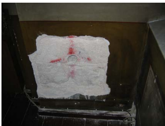
Figure-5: Area without mortar cover
