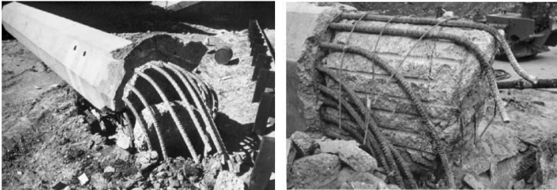
Figure 1: Pull-out of longitudinal reinforcement in bridge columns from foundations during the San Fernando (1971) earthquake [1]
