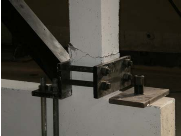
Figure 17: Plastic hinge at the bottom of the column (F1)
