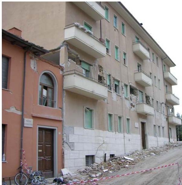
Figure 1: Damage of a four-story conventional building due to pounding with its adjacent two-story building, during the L'Aquila earthquake in Italy, in April 2009
