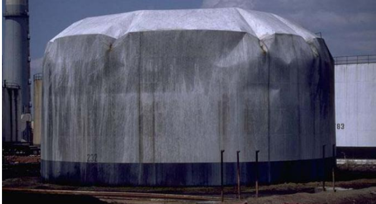
Figure 18: Sloshing buckling at the top of a tank; Kocaeli, Turkey earthquake 1999 [1].
