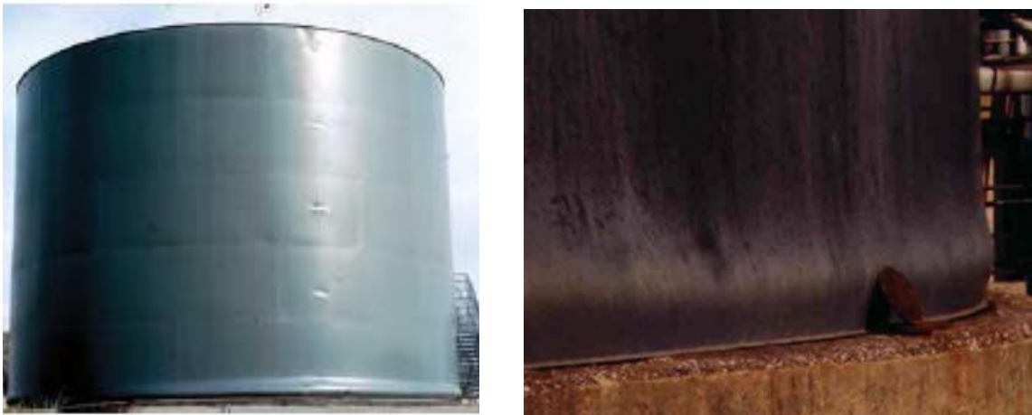
Figure 14: Elephant’s foot buckling caused by strong earthquake action.
