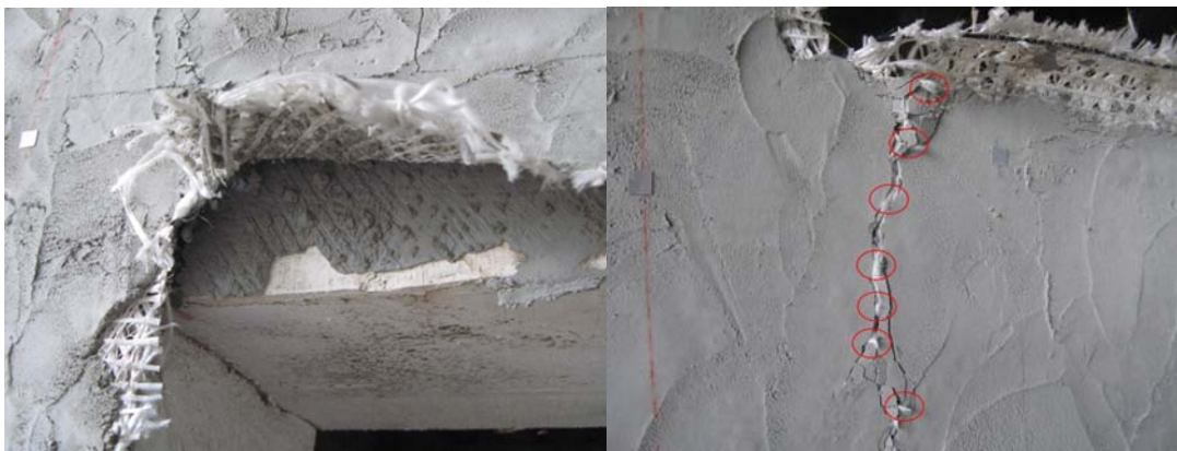
Figure 10: Crack pattern: a) delamination, b) broken glass fibers
