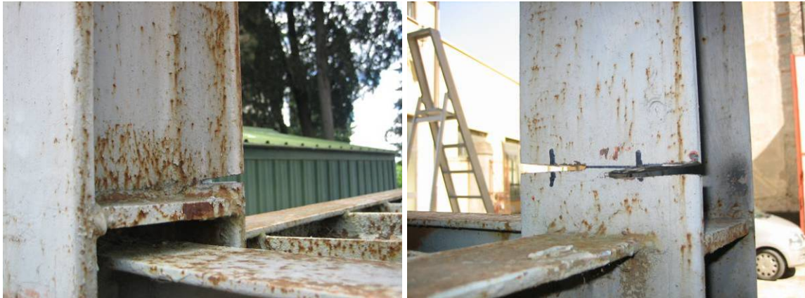
Figure 3: Damage Level #1 (left) and Damage Level #3 (right).
