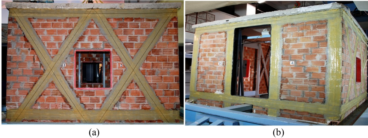
Figure 8: A picture of the repaired masonry building with reinforced GFRP strips; (a) sides 1-2, (b) sides 3-4.
