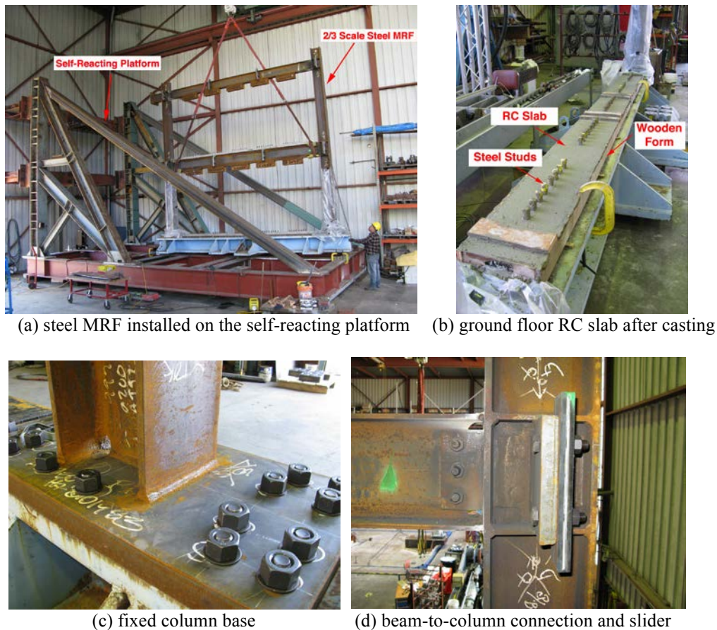
Figure 4: Erection and typical connection details of the physical subassembly part of the hybrid model.
