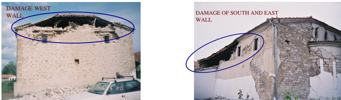
Figure 17. Representative damage patterns of the “Typical Basilica”
