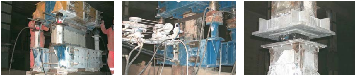
Figure 7: Phases of the retrofit of the building of Figure 6, with installation of 4 hydraulic jacks to provisionally support the weight after removal of the pillar part to be replaced by an isolator and to locally lift the building, so as to allow for the subsequent insertion of the isolator (left), and cut of the pillar with a linear saw (at the centre); view of the isolator after its installation and its mechanical fixing to the upper and lower pillar parts (right).
