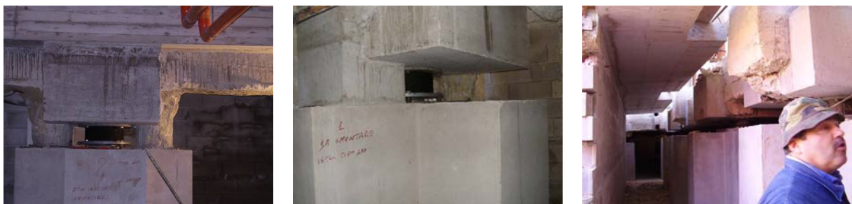
Figure 18: HDRBs installed between two original (left) and two newly built (at the centre) foundation piles of the house of Figure 11, before demolition of their parts which were not encompassed by the new pillars; the underground floor after demolition of the aforesaid parts (right).
