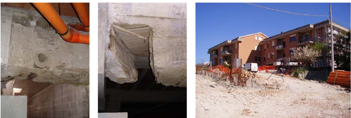
Figure 20: Holes and breaks in the beams of the house of Figure 11, made during the initial construction to create passages for the pipe lines (left and at the centre); the house after retrofit completion (right).
