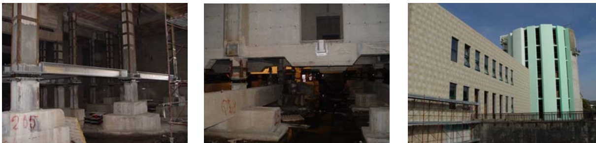
Figure 8: Installation of the steel beams floor in the building of Figure 6 just above the isolators and reinforcement of the pillars (left); the lower floor after cut of the building supporting pillars and walls (at the centre); the building after retrofit completion (right).
