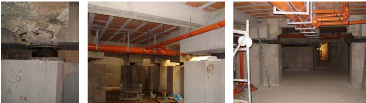
Figure 19: A HDBR installed, after demolition of the parts of the original foundation piles which were not encompassed by the new pillars (left); the new underground floor in the aforesaid conditions and after the installation of the pipe lines (at the centre and right).
