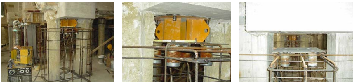
Figure 15: Setting up of the reinforcement of the lower stump of the new pillar (by means of a dummy isolator) and of the lower plate for connecting the isolator in the new underground floor of the house of Figure 11.
