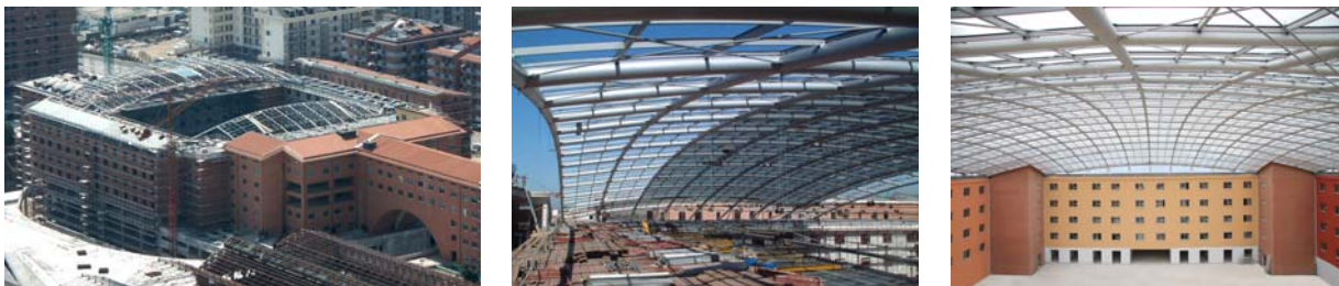
Figure 22: New ceiling of the Crowne Plaza Hotel in Caserta, set up by the GLIS board member and ASSISi member G.C. Giuliani of Milan in 2006 by constraining it by means of SDs to 3 of the 4 buildings to which it is connected.
