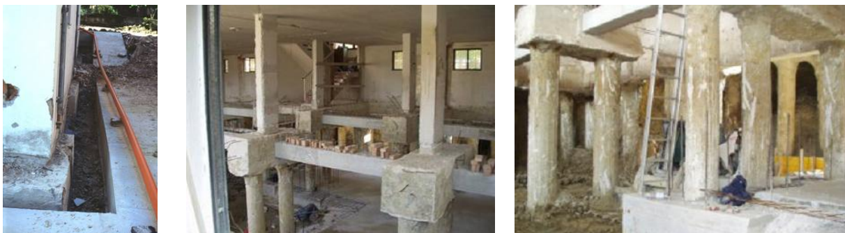
Figure 13: Creation of the structural gap around the house of Figure 11 (left); view from the top of the original lower floor and the new underground one after excavation of the latter and construction of new curbs (at the centre); view from the bottom of the new underground floor, the original foundation piles and the new foundations under constructions (right).
