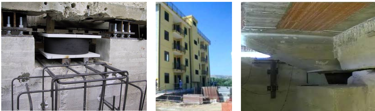
Figure 10: A HDRB during its installation in one of the buildings of Figure 9 (left); this building after retrofit completion (at the centre); an isolator laterally deformed during the on-site tests (right).
