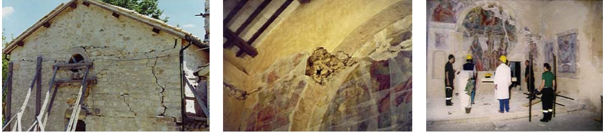
Figure 24: External and internal damages suffered by the San Giovanni Battista Church in Apagni (Perugia) during the 1997-98 Marche & Umbria earthquake.
