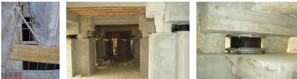
Figure 17: Lateral structural gap of the house of Figure 11 before the installation of its protection plates (left); the new underground floor after installation of the HDRBs, but before demolition of the parts of the original foundation piles which were not encompassed by the new pillars (at the centre); an installed HDRB superposed to an epoxy flat jack (right).
