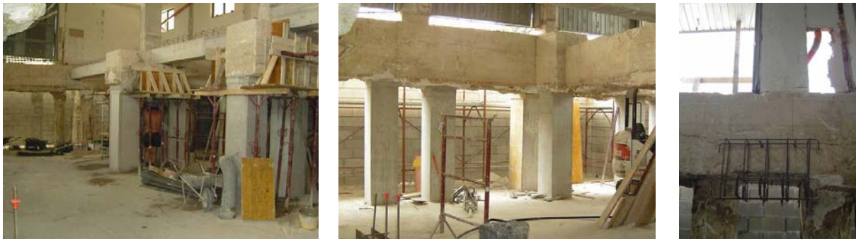
Figure 14: Newly built foundation piles, in the part of the house of Figure 11 where the original ones were failing (left and at the centre); pillar eccentric with respect to the original foundation piles (right).
