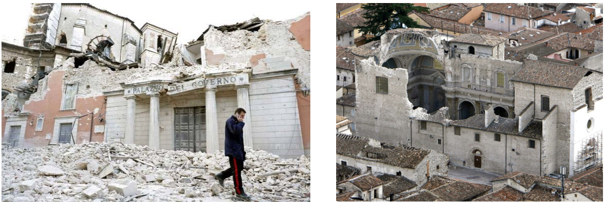
Figure 3: The Prefettura building (provincial headquarters of the national government) of L'Aquila, a symbol of lack of prevention of the seismic risk in Italy until 2009 (left), and the Santa Maria Paganica Church (right), collapsed after the 2009 Abruzzo earthquake.
