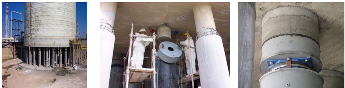
Figure 23: One of the 3 tanks of Polimeri Europa located in Priolo Gargallo (Augusta, Syracuse, seismic zone 2*), which were seismically retrofitted using U.S. FPS devices in the years 2005-2008 and one of the isolators during and after its installation.
