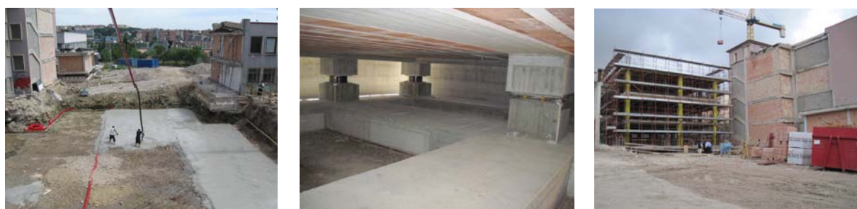
Figure 39: The Romita High School in July 2010, after the demolition of blocks “A” and “B” (left); two HDRBs and a SD installed in the underground technical floor of the new block “B” of the school, during its reconstruction (at the centre); state of the reconstruction of the new block “B” in October 2010, before casting of the upper deck, at the side of the original block “C” (right).
