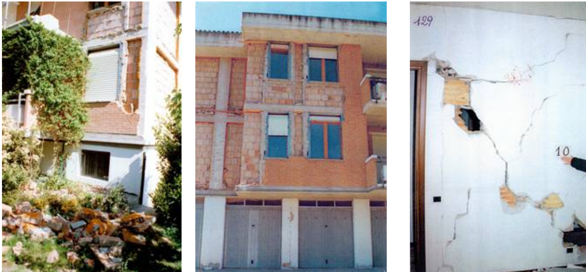
Figure 12: External and internal non structural damage suffered by the house of Figure 11 in the 1997-98 Marche & Umbria earthquake.
