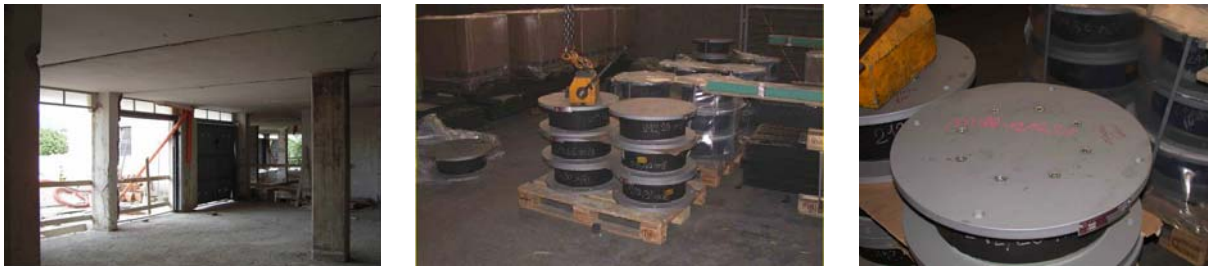
Figure 16: New r.c. slab of the ground level floor of the house of Figure 11 (left); the HDRBs before their installation in the new underground floor (at the centre and right).
