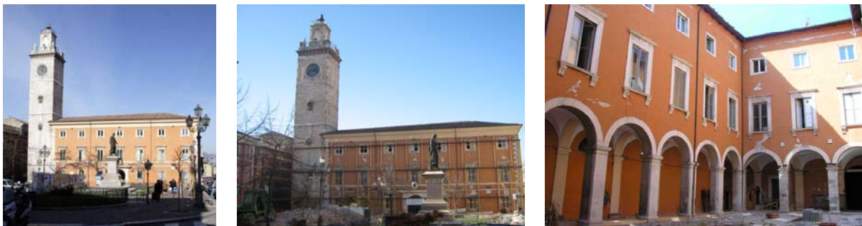
Figure 36: The monumental building Palazzo Margherita in L'Aquila before the 2009 Abruzzo earthquake (left) and put in safe conditions because of the damages suffered during this event (at the centre); its internal courtyard after the earthquake (right).
