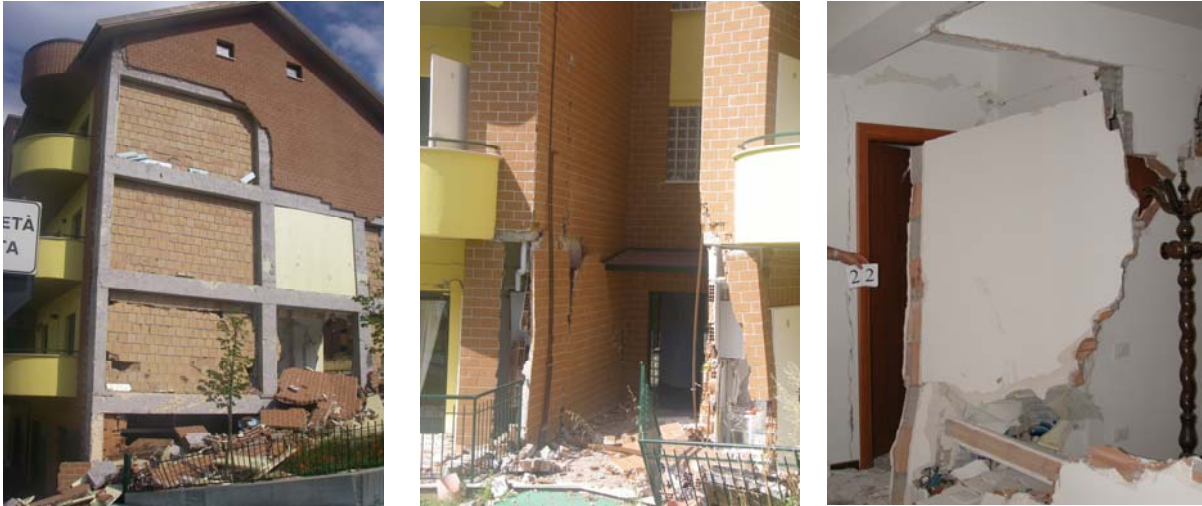
Figure 35: Damage caused by the 2009 Abruzzo earthquake to the building of Figure 34; its retrofit by means of HDRBs and SDs has been planned, based on a design of the already mentioned GLIS and ASSISi member G. Mancinelli of Fabriano, with safety certification of A. Martelli.
