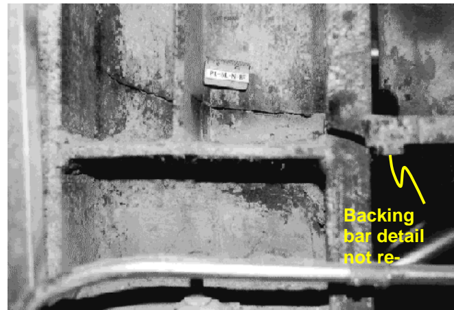
Figure 1: Fractured connection in a steel moment frame during the 1994 Northridge earthquake (crack propagated at backing bar detail and propagated in the column flange and web)
