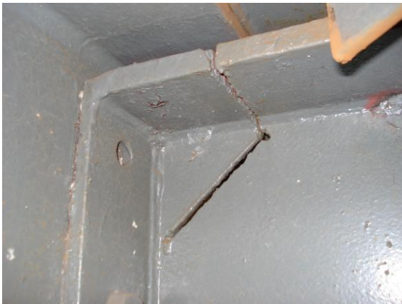
Figure 12: Typical fatigue damage and repair of track bracing cross beams
