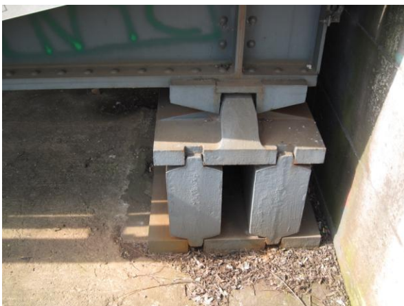
Figure 10: General view of unidirectional bearing
