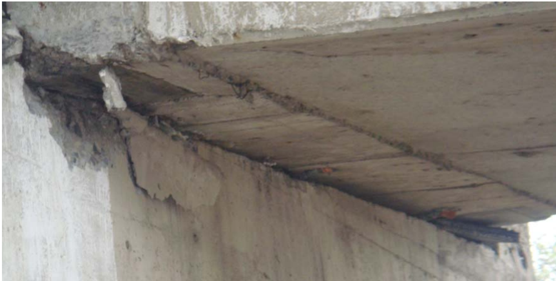
Figure 1. Relative response induced damage of Puente Llacolen in the 2010 Chile earthquake
