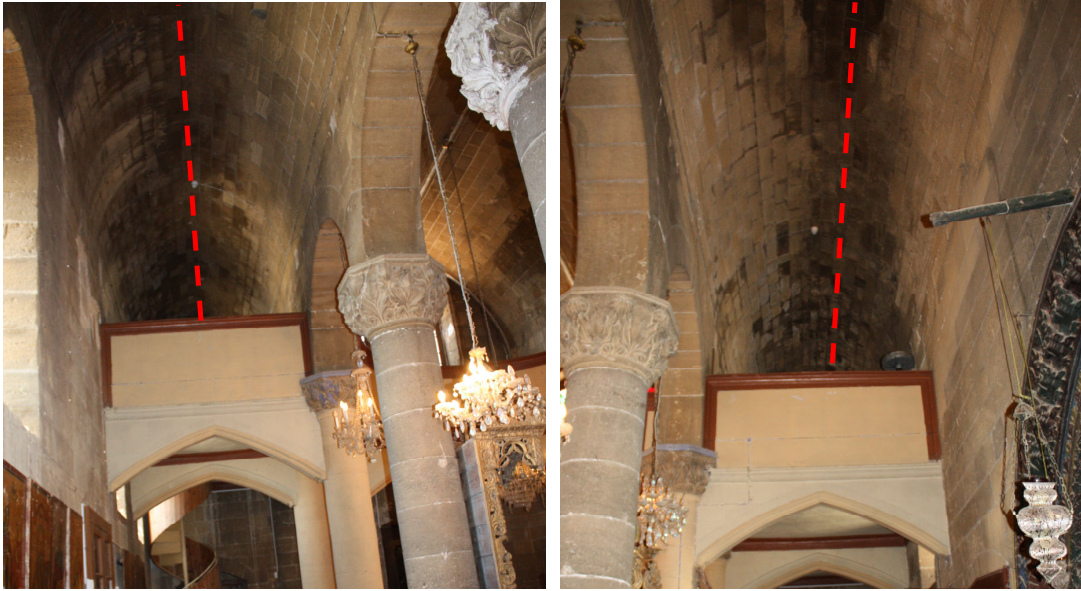
Figure 2: Pictures depicting two aisle vaults along which the lowest temperatures within the structure were detected.
