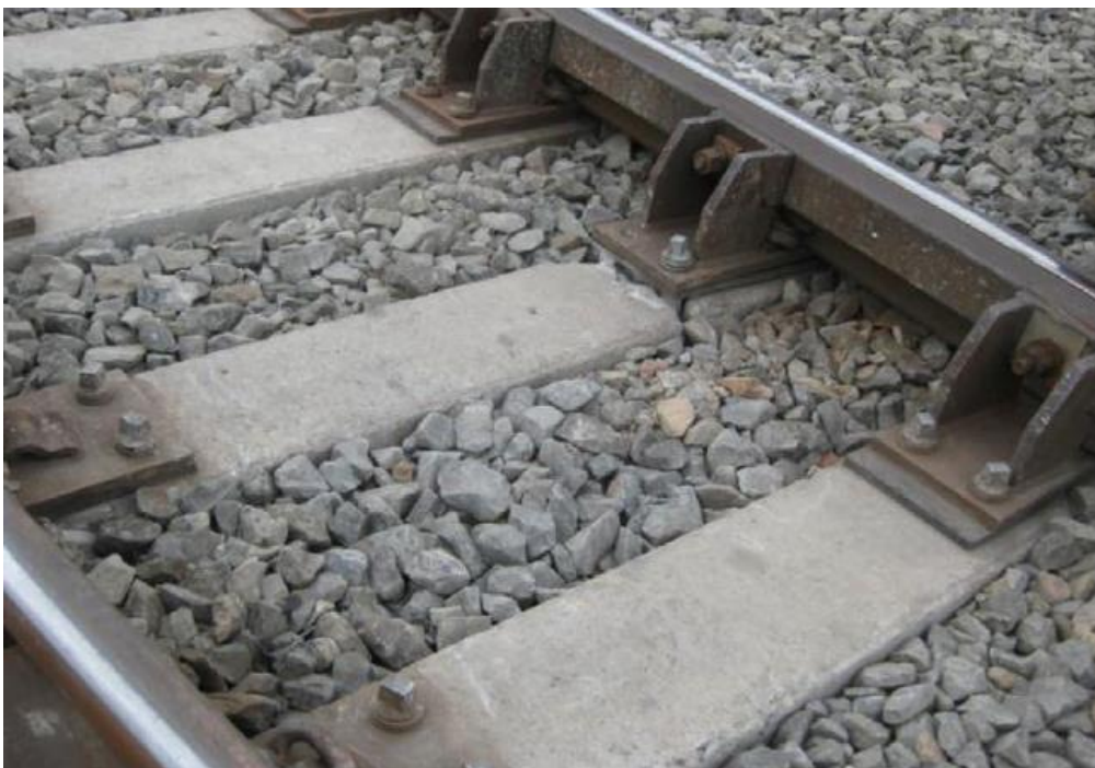
Figure 6: Evidence of a failure mode of concrete bearer found in the field [35].
