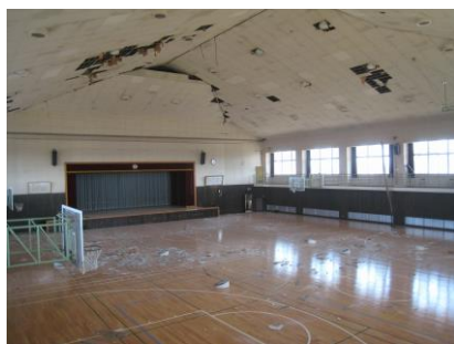
Fig.1 Ceiling collapse occurred in a school gymnasium
