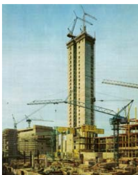
Figure 1: Building under construction in 1971 and erection of the transfer beams painted in yellow.
